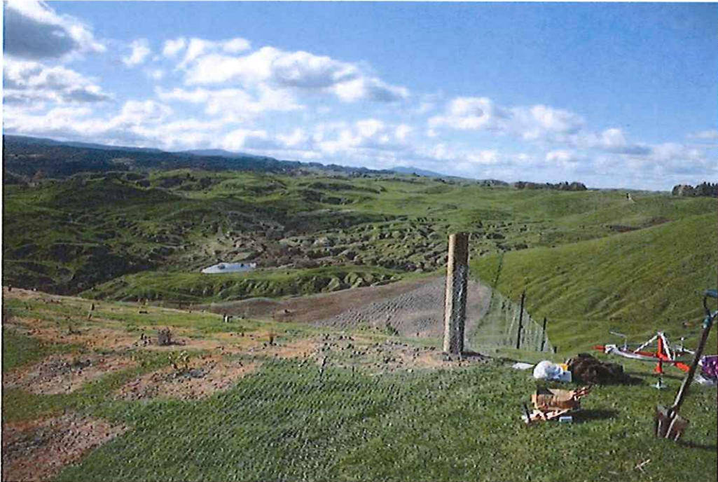
Figure 7: Construction of the rabbit proof fence around the trial area to prevent rabbits, hares and livestock from entering the site at Waihaha, west of Lake Taupo.
